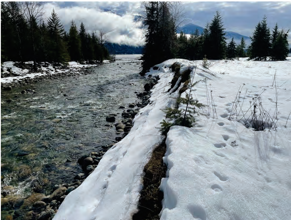
Photo 4: Looking downstream at right bank erosion
