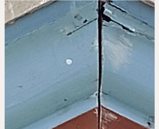
Damaged Historical Detailing
