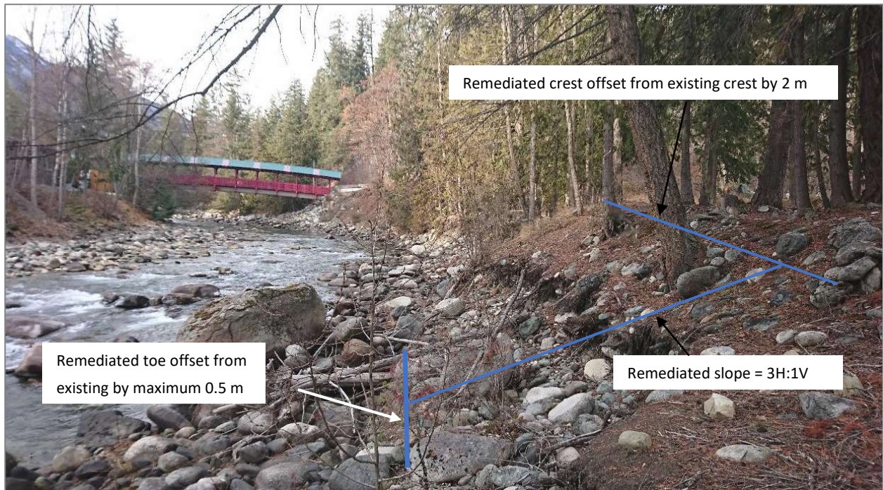
Photo 5. Upstream view of riverbank within Lot A showing general design of proposed scour protection.
