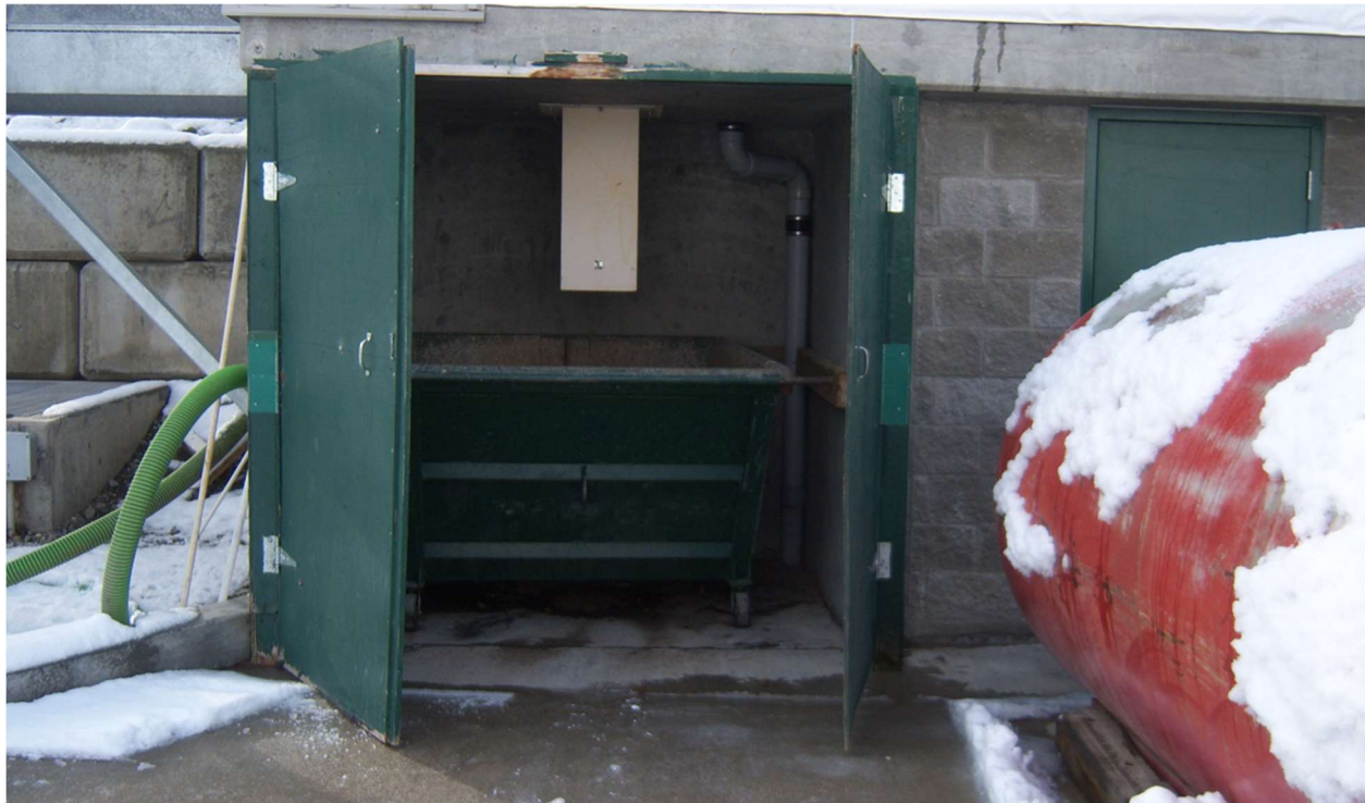
FIGURE 4-4: WASTE BIN LOCATED BELOW SALSNES™ FILTER (LILLOOET, BC)
